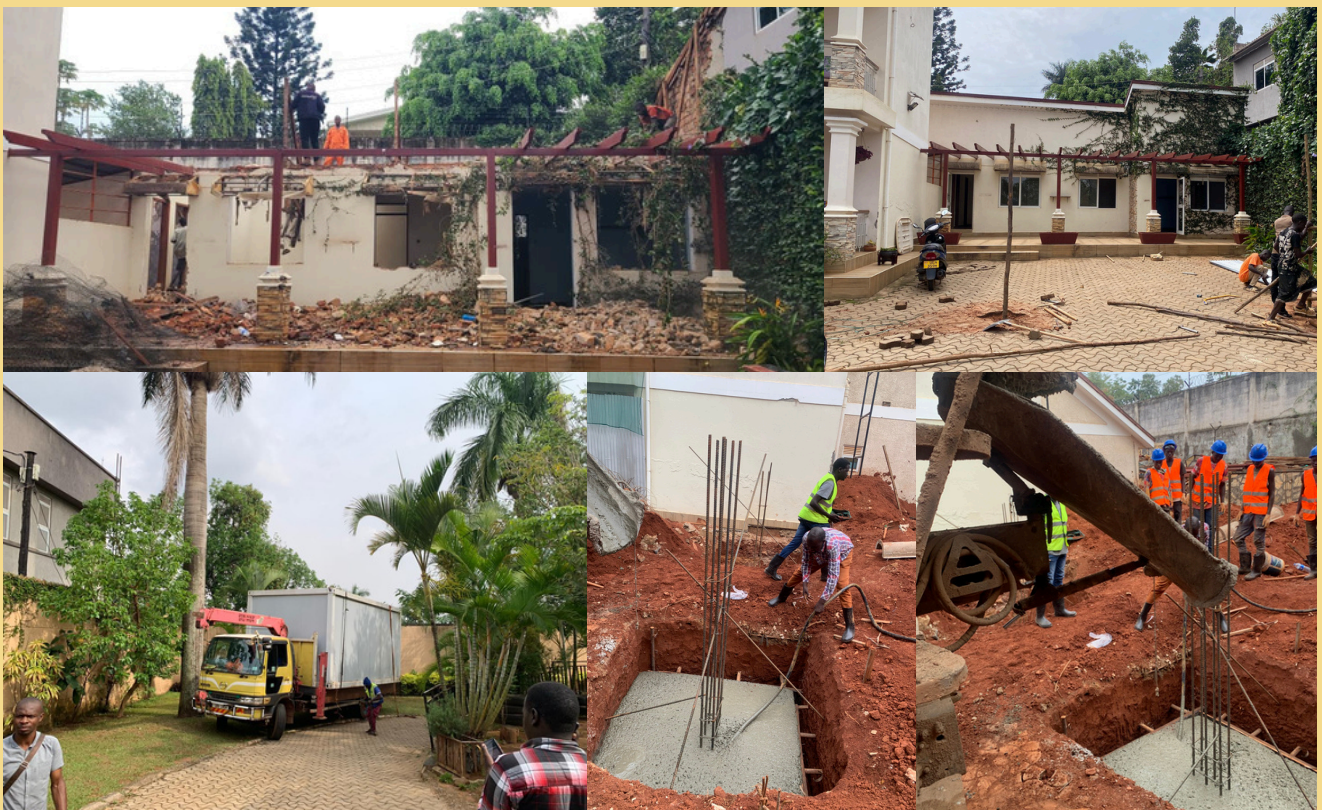
Brook House reconstruction began steadily although its been rainy season the workers is progressing.
